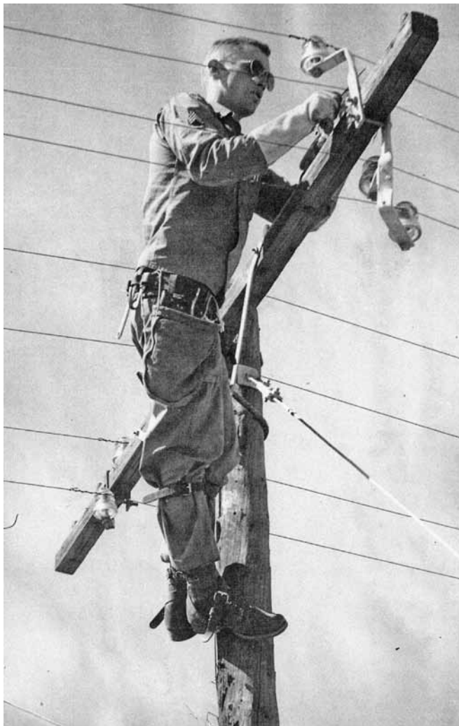
Sergeant Johnny Lay up a pole tying in open wire communication lines at White Sands in 1952.
