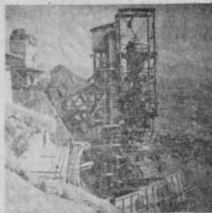
READY TO ROAR — With the Redstone motor anchored into place beneath cylindrical fuel tanks, the final modification of the 500 K test stand is complete and ready for firing. The huge tanks, which contain fuel and oxidizer propellants, to run captive Redstone motor, are specially designed for research and development purposes.
