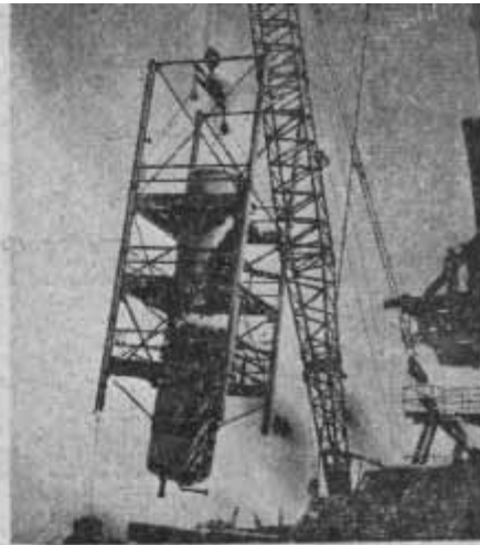
THE BIG LIFT — A 45-ton crane heists the Redstone propellant tank cage into a vertical position at the 500 K. Workmen welded the Redstone modification onto the stand to enable the Redstone missile motors to be tested at the stand. The cage and fuel tanks weigh an estimated 30 tons.
